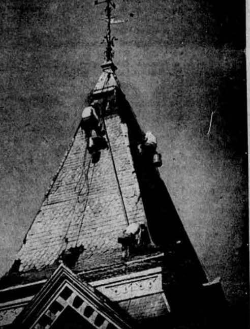
ANOTHER SHOT—The above picture was made from in front of the fire station, using a 15-inch telephoto lens. It shows a close-up view of workmen putting on the new roof. Work is still underway with them using a paint-job being applied.
