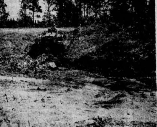
HOMER LANIER of the Statesboro Sanitation Department is shown here as he operates the new bulldozer which is the key to the new land fill method of garbage and trash disposal. The new method assures the city of a safe and sure and sanitary means of protection against garbage odors, flies, and rat infestation at the garbage disposal site.
