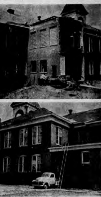
TOP PHOTO shows the old Statesboro High School Building on South College Street in the process of being renovated to provide additional classroom space for the Statesboro School. The section with openings will be torn away from the main building. The bottom photo shows the north side of the building where repairing on the roof is being done. The picture shows the windows of the second story being boarded up. This building was erected at the turn of the century. In 1923, the new high school building was completed on West Grady Street and this building became the grammar and elementary school. —Herald Photo
