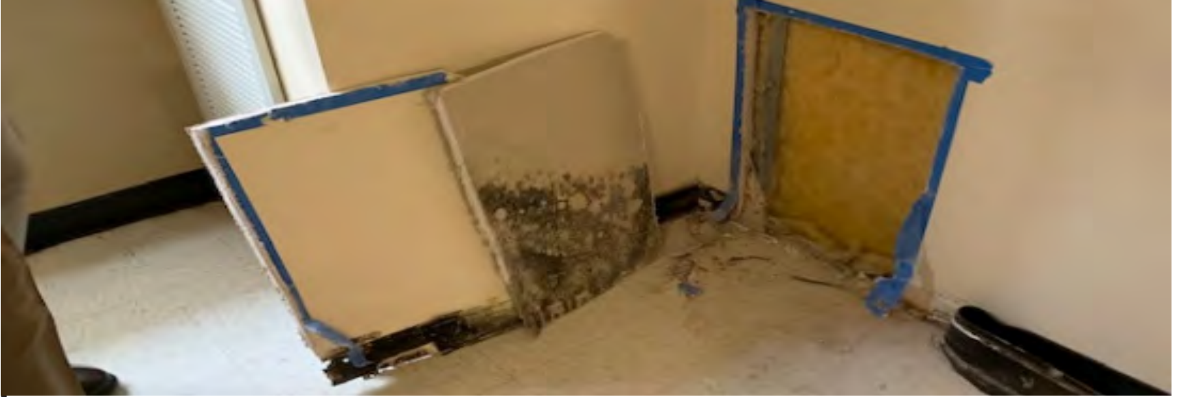
PHOTO COURTESY OF Mold Investigation Documents
