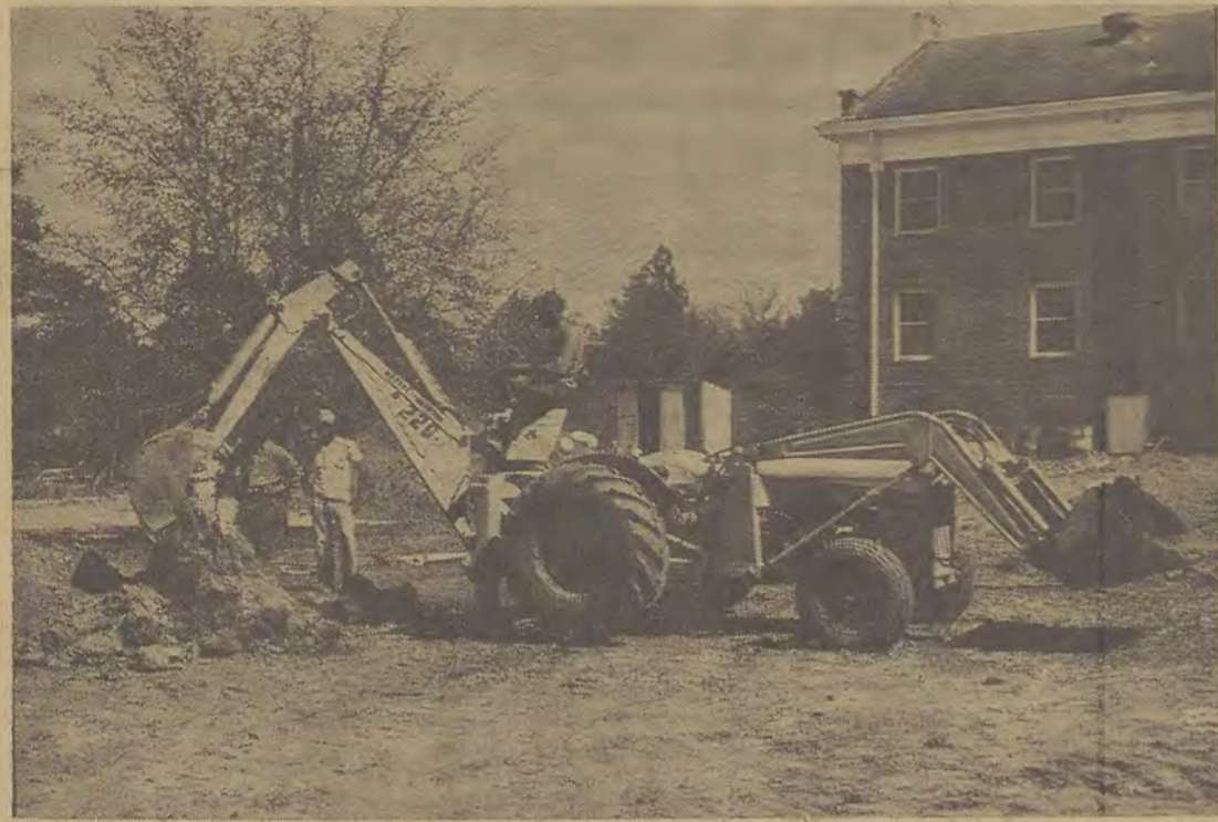
WORK IS UNDERWAY! This was the scene behind Lewis Hall Tuesday as ground was broken for the construction of an annex there. The Lewis Hall Annex, when completed, will house 78 GSC women. It will contain 26 rooms plus a house director's apartment and activity room.
