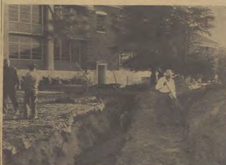
WORKERS ARE SHOWN here as they continue construction of the new college sewage system. Construction, which began in late summer, is expected to be completed by November 1. This is the third and final phase of the new system which is being constructed on the west side of the campus.
