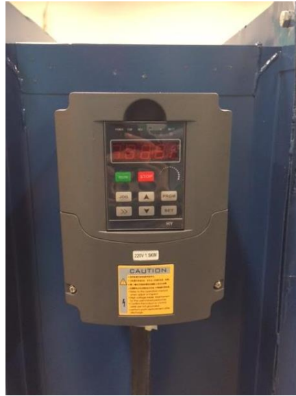
Figure 3.13. Huanyang Variable Frequency Drive Operator Interface
