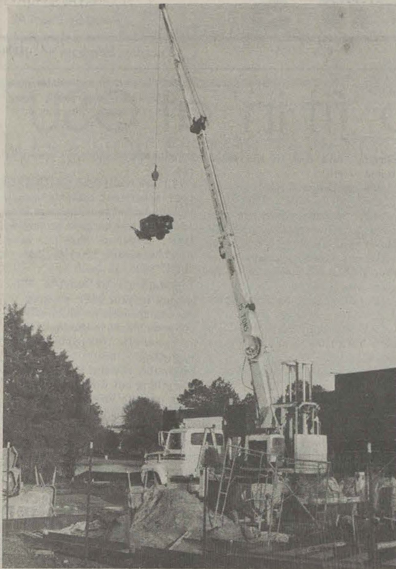
Swingin' in the breeze: Not even 7-foot tall Eagles hoopster Emmett Smith could reach this welder. (Photo by Clint Home.)
