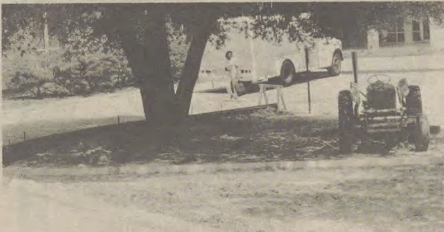
GSC will soon have a new park, complete with benches, in the area between Rosenwald, Hollis and Herty. Construction should be complete by May 20.
