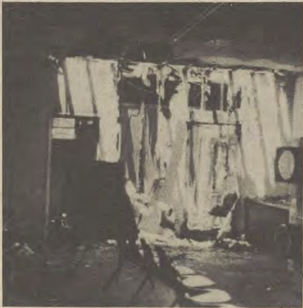
The In-the-Pines clubhouse caught on fire May 14. The state fire marshall has not yet determined the cause of the fire, but Director of Auxiliary Affairs Larry Davis said the cause may have been an electrical short. Davis estimated the cost of damage to be around $10,000. Davis anticipates the clubhouse will be opened again in the fall.
