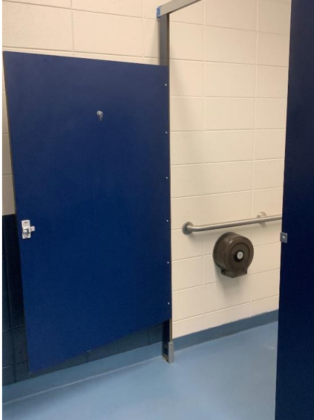
Figure 1. Bathroom stall that makes it difficult students for independent restroom use.
