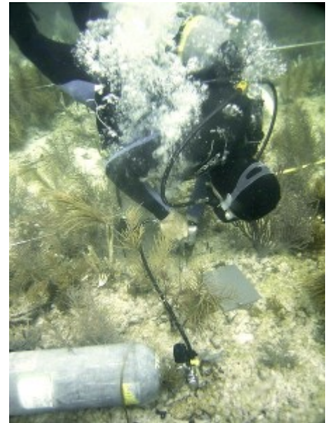
Danny Gleason, Director, ICPS, uses a pneumatic drill connected to a scuba tank to create a small hole in the reef. A drywall anchor and stainless steel bolt will be installed in this hole.
