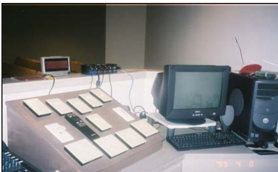
Dimmer switches and computer.
